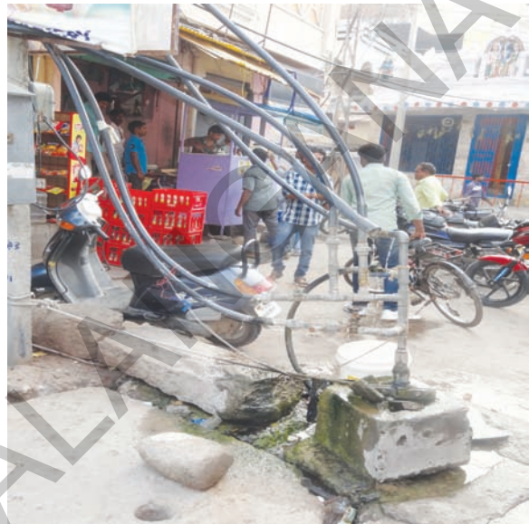
Fig. 14.6: Pipe lines for drinking water(Akasha Ganga)
